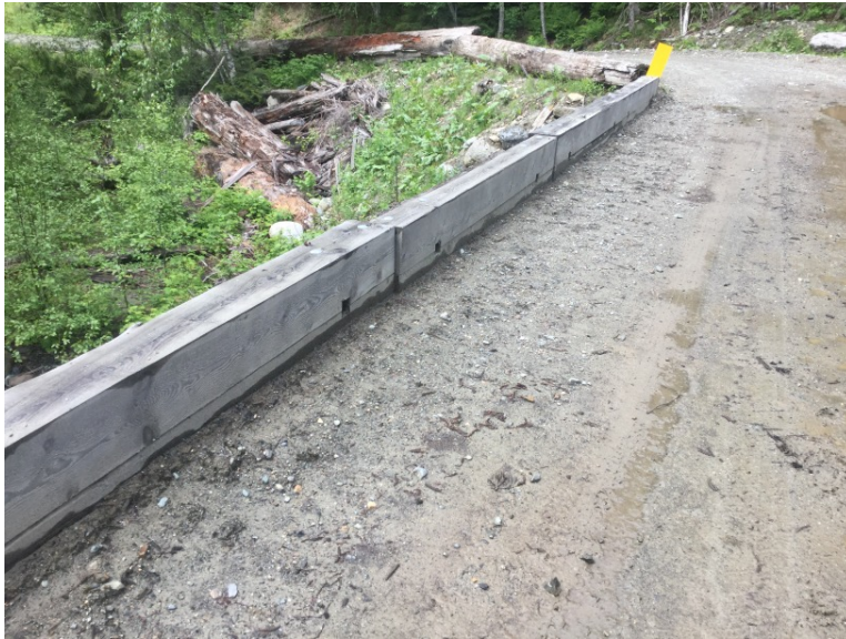
Full riser with drain holes
